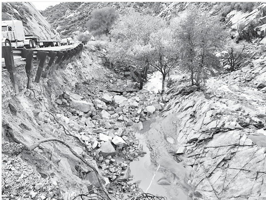
Flood damage to U.S. 60 between Superior and Miami following recent monsoon rains. Photo Courtesy ADOT
