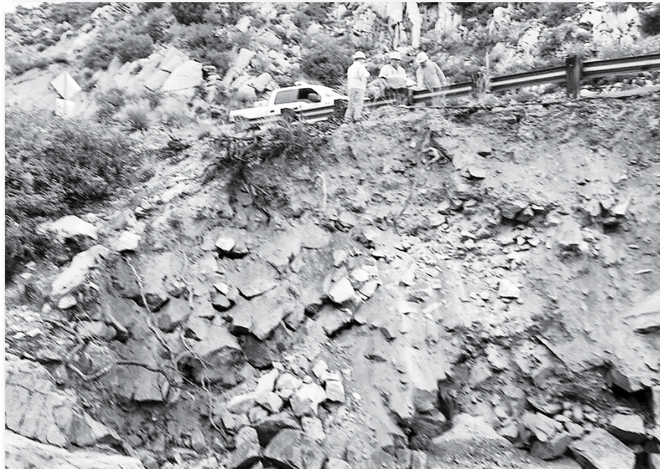
Flood damage to U.S. 60 between Superior and Miami following recent monsoon rains. Photo Courtesy ADOT
