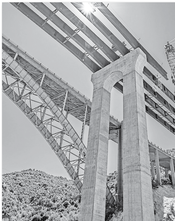
ADOT has announced a week long road closure as they prepare to reroute traffic onto the new bridge at Pinto Creek. Photo courtesy ADOT
