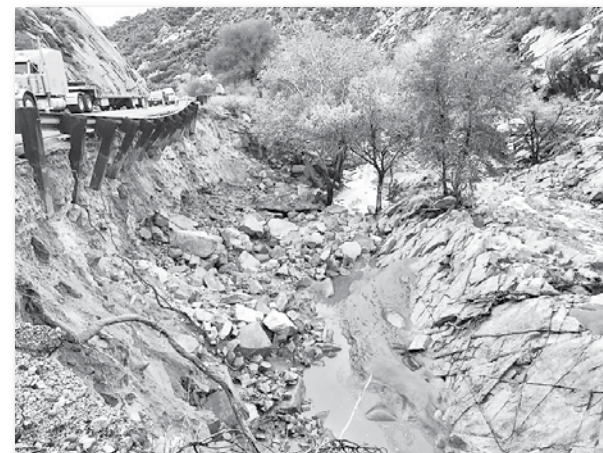
Flood damage to U.S. 60 between Superior and Miami following recent monsoon rains.
