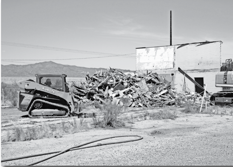
This motel in Hayden was demolished by Gila County with financial assistance from a brownfields grant.
