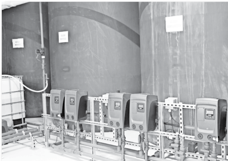
Part of the water recycling system at the Flower Mine in San Manuel.
