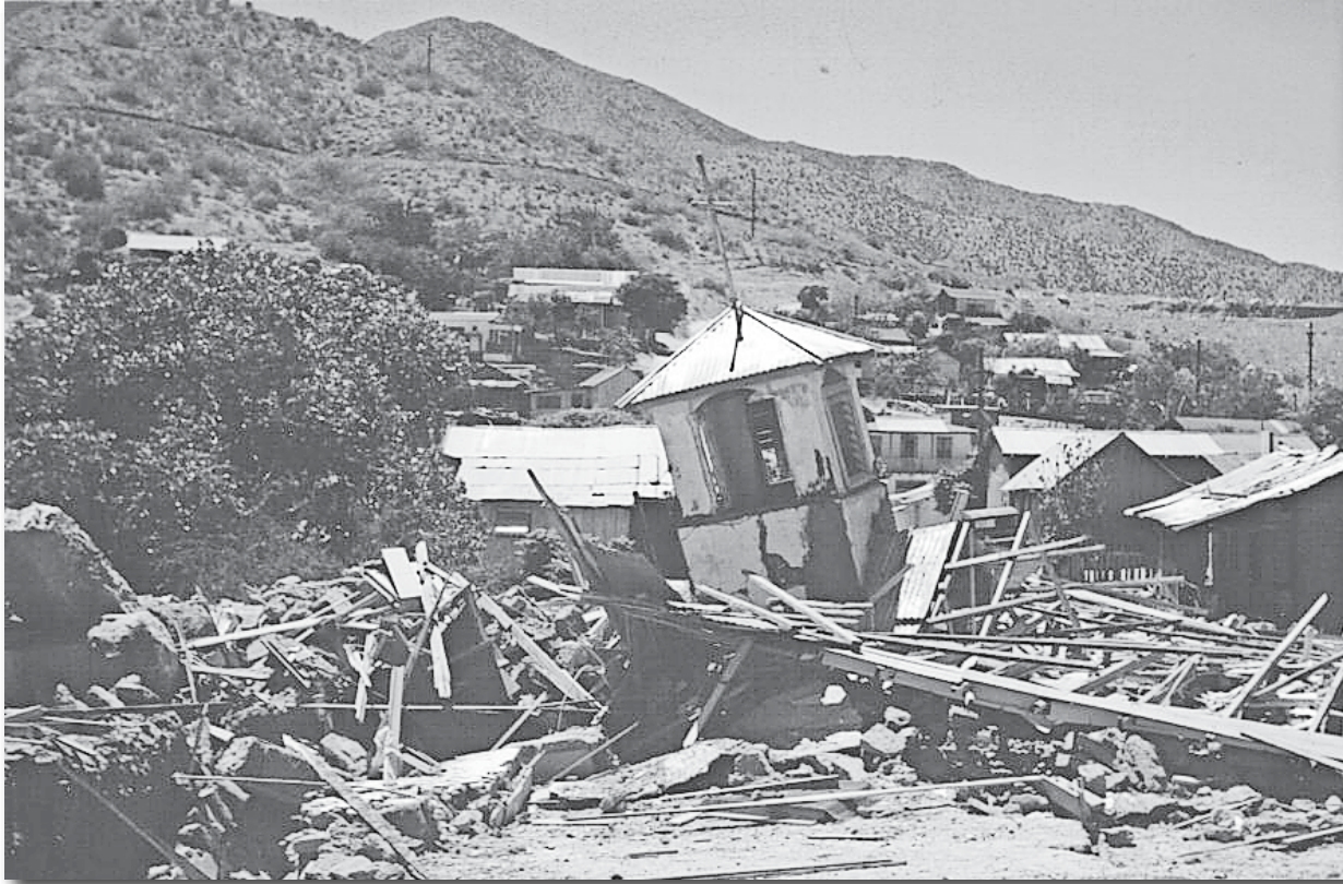
Demolition of the St. Helen's Church not moved to the new site in Kearny.
