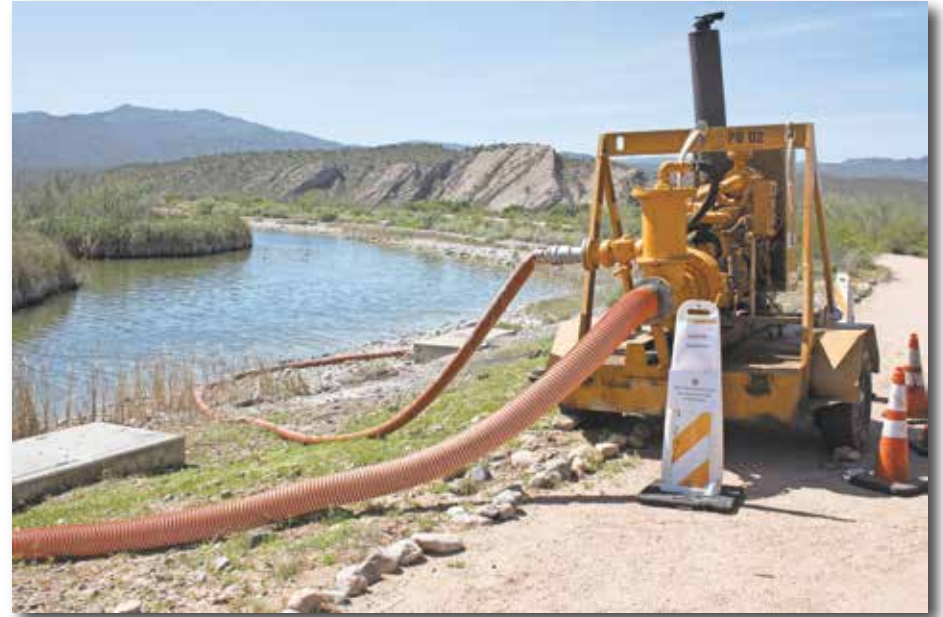
Draining the Kearny Lake is part of the lake repair. Water is being pumped out of the lake and into Steamboat Wash. James Carnes | CBN
