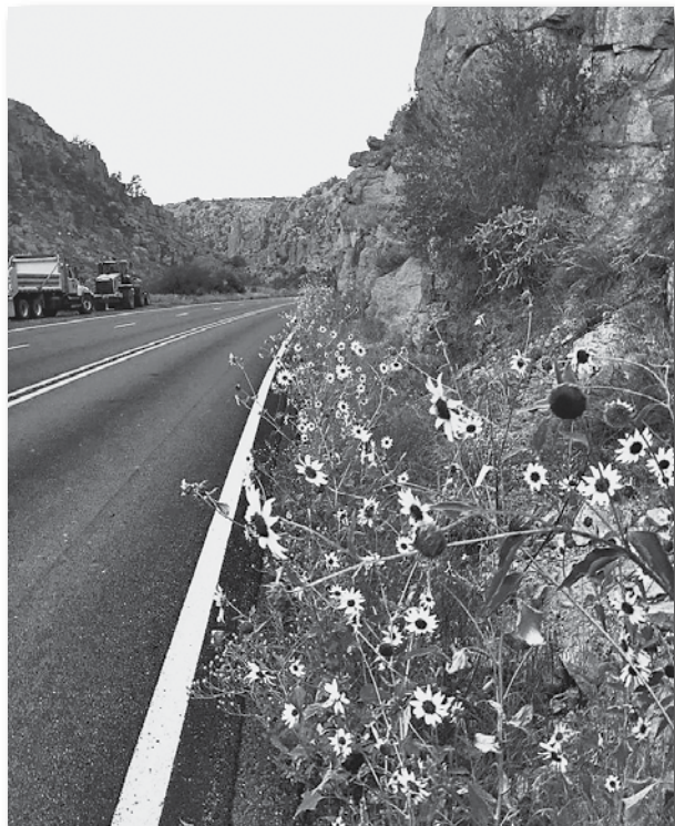
US 60 before (left) and after (right) the clean up during the closure.
